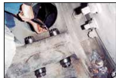
Split gear segment on rotary kiln.
