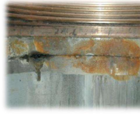
Crevice Corrosion (narrow Clearances)
