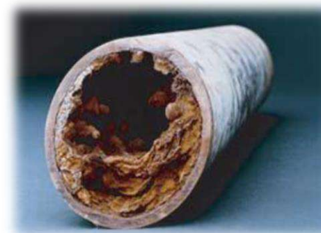
Erosion Corrosion (Microbiologically Induced corrosion)
